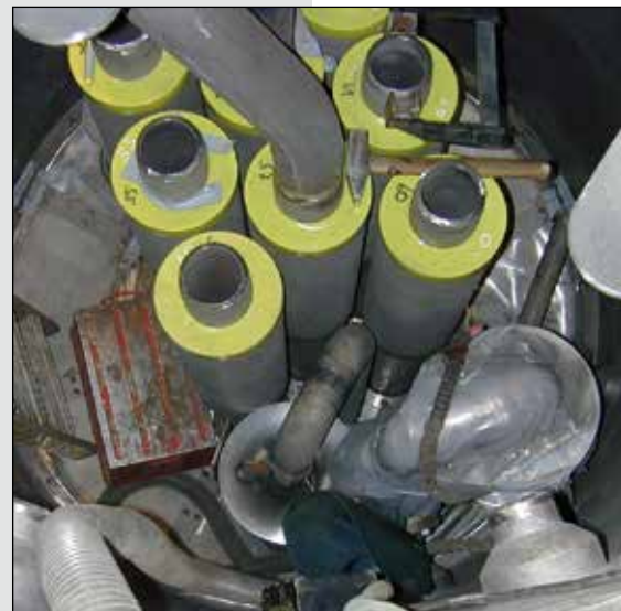
View from above on injector and connecting tubing to double tubes
